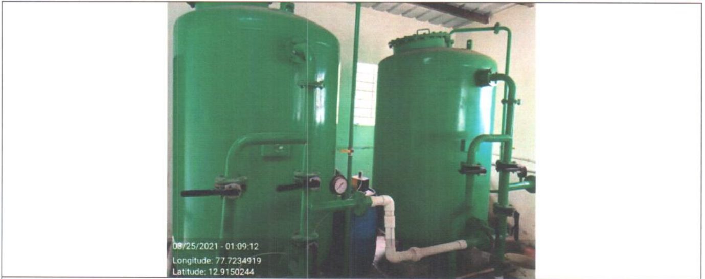
STP unit for waste water recycling
