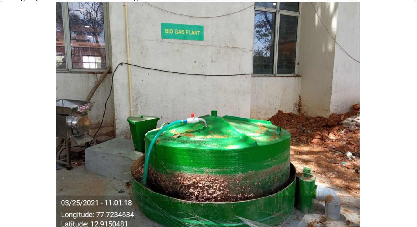
Bio gas plant for solid waste management
