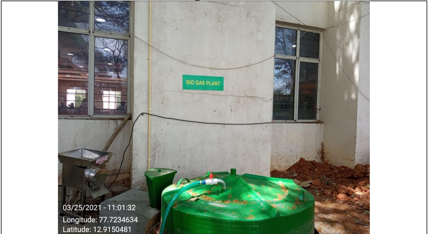
Bio gas plant for solid waste management
